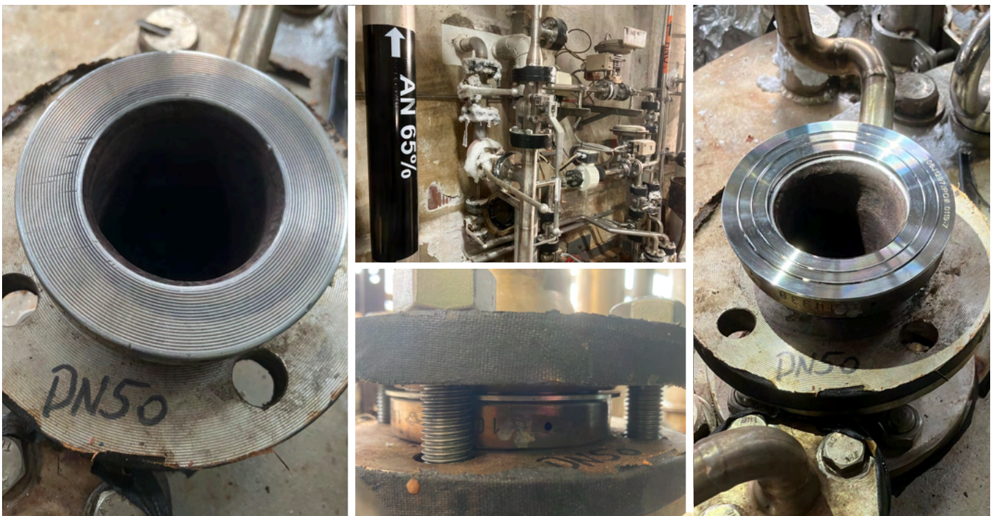
Left: DN50 flange, prior to install (note light scoring marks) Top Centre: Overview of area where DeltaV-Seals to be installed. Bottom Centre: DeltaV-Seal Installed Left: DeltaV-Seal mid-installation.
