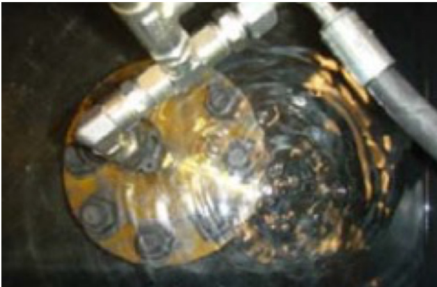
Figure 17. Helium testing - 5 barg - Leakage up to 95 Nm torque
